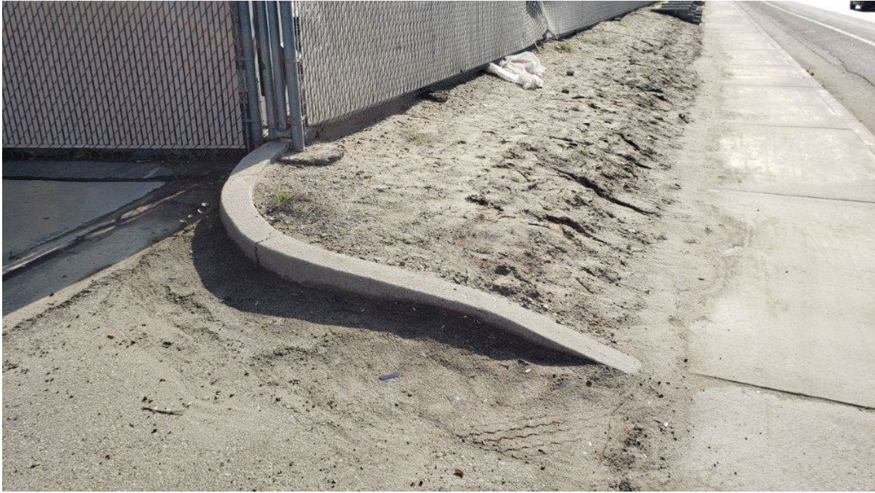
South entry – south side condition
