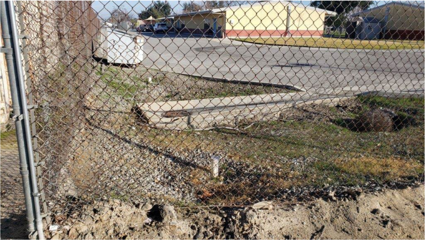
KCSOS sump requiring re-grading, rock and weed barrier.
